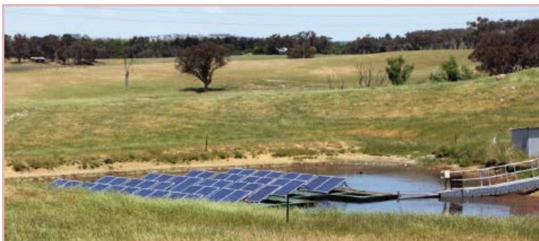
Figure 13 Floating solar array (NSW Farmers, 2015b).
