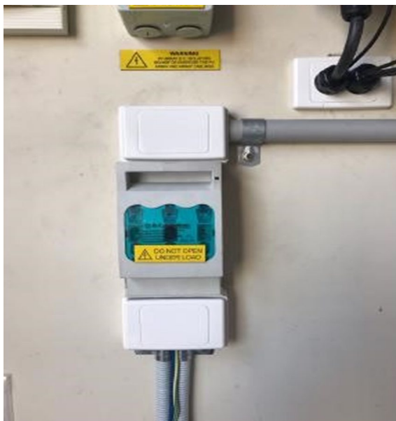
Figure 16 Rectified wiring after compliance and conformance inspection
