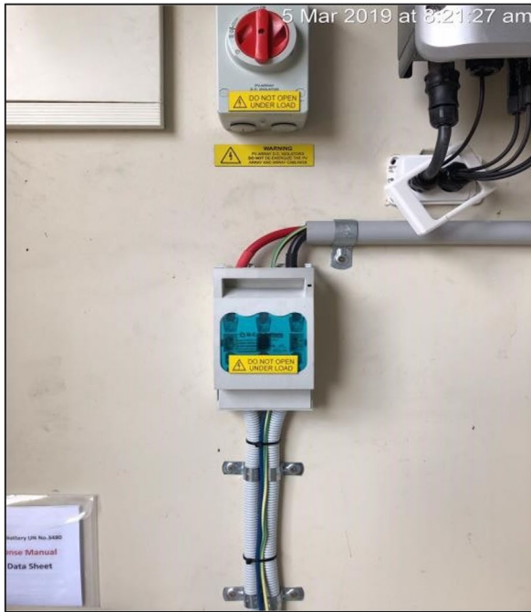
Exposed LIVE parts
