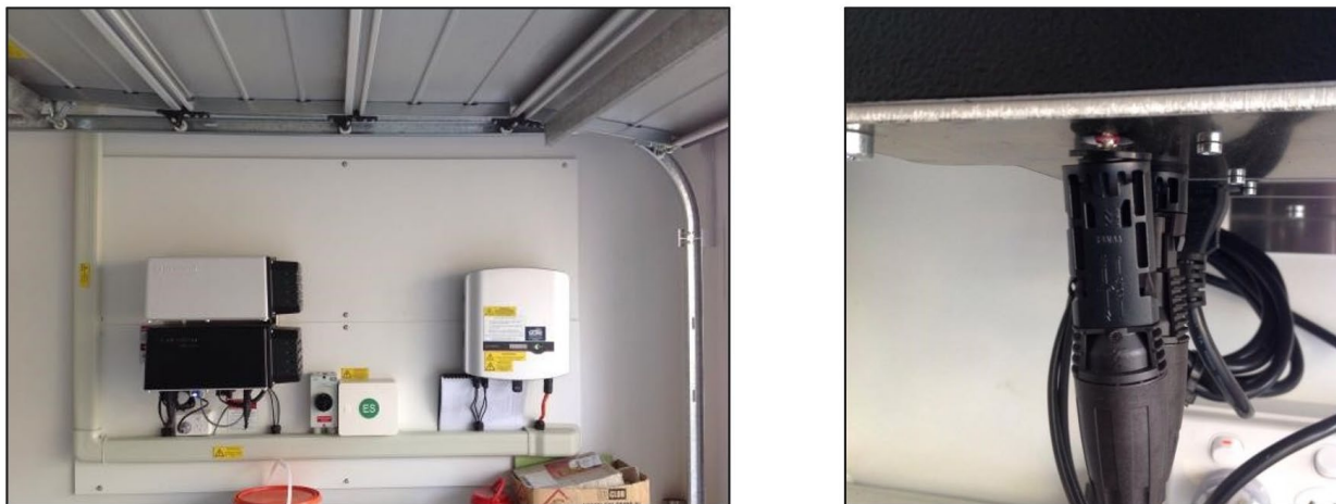
Figure 17 Observation of a battery installation with damaged plug and exposed conductors
